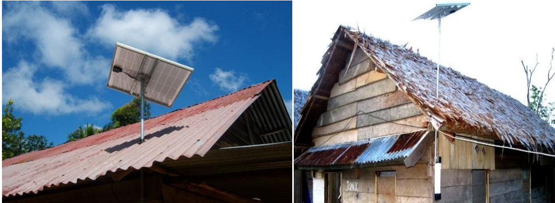
Fig 4. Implementation of Solar Home System on Vilages.
